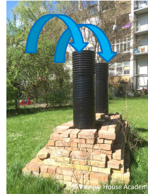
Intake tubes for earth tube pre-heaters
