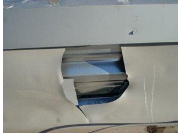
Damage of waterproofing membrane caused by UV radiation
