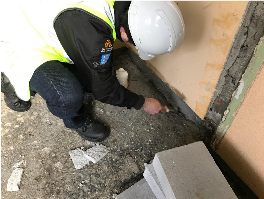
Floor to wall junctions, where surfaces are rough and preparation is essential
