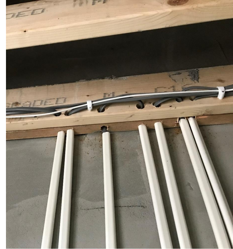
Multiple services passing through wood without special airtight grommets
