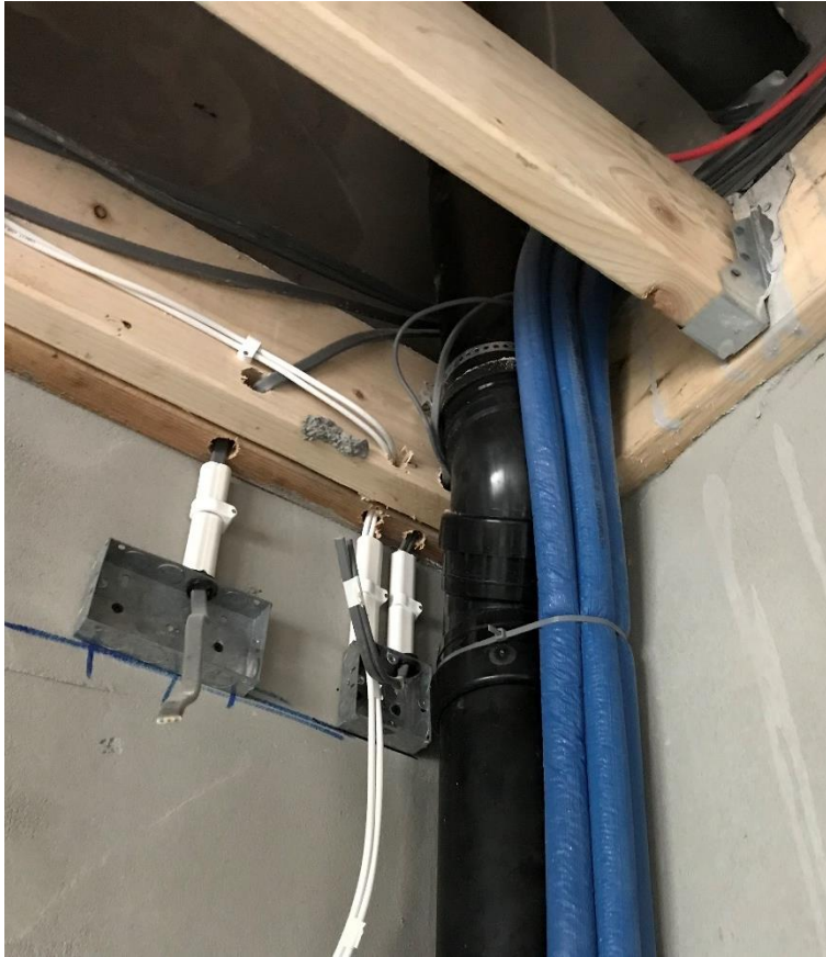
Bunched service penetrations fit tightly to corners which cannot be individually taped or sealed
